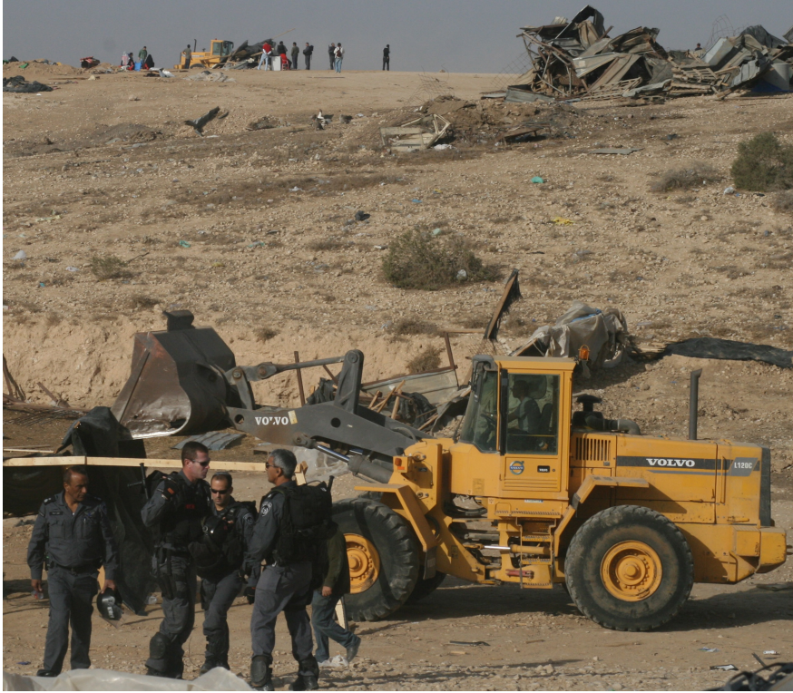
Figure 3: Bedouin House Demolition in Beersheba Region, 2018 (Photo: Negev Coexistence Forum by permission).
